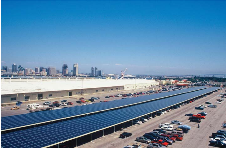
Figure 1. U.S. Navy 750 kW Parking Lot Solar PV Installation near San Diego.
